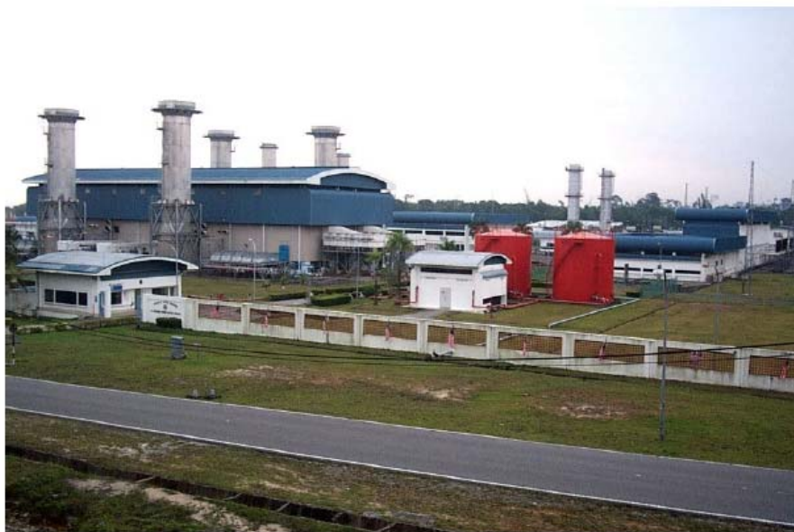
Existing Gas Turbine Generator Sets
